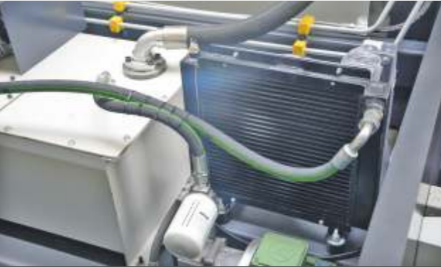
Hydraulic Oil Cooling System
